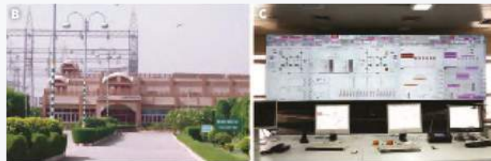
Fig. 2 - Front view and control room of Bhiwadi substation
